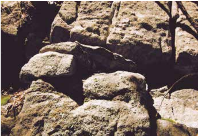
Crumbling and excessively fractured rock face
